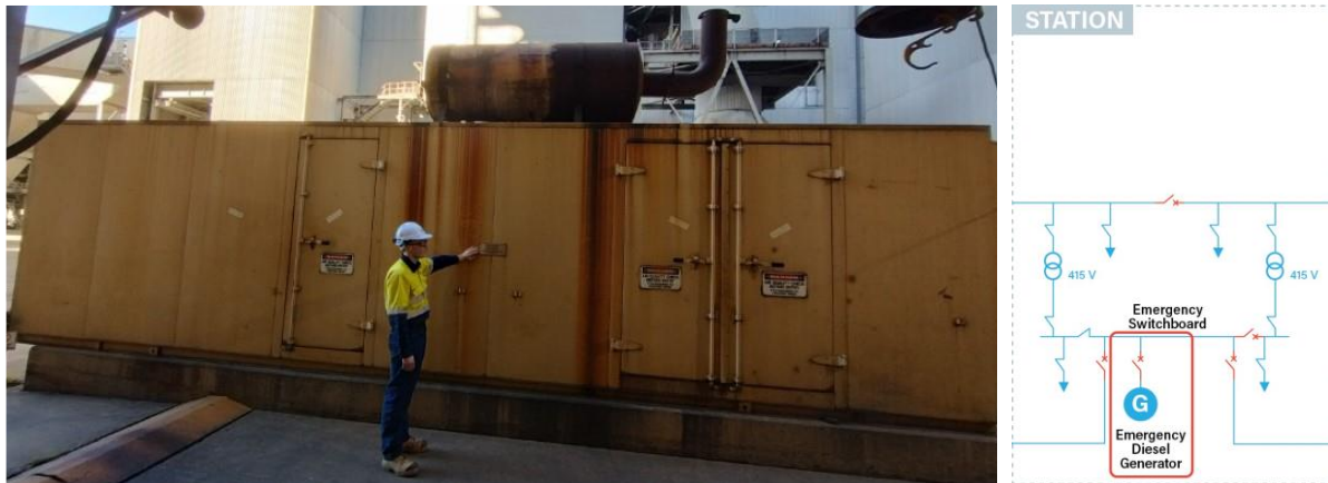
Figure 57 Emergency diesel generator
