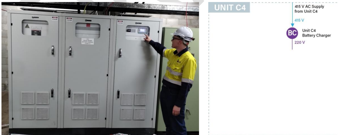
Figure 60 Unit C4 battery charger
