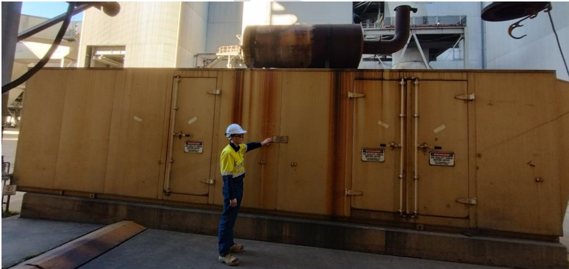
Figure 19 Unit C4 emergency diesel generator
