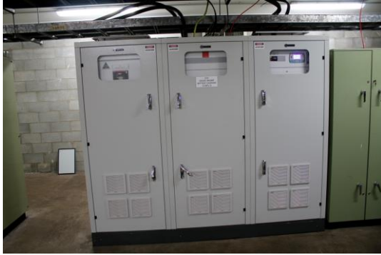
(a) Unit C4 battery charger
