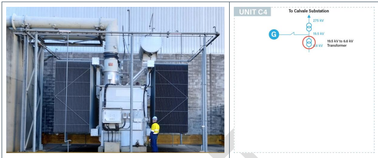
Figure 47 Step-down transformer (circled in red)
