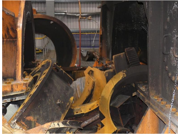
Figure 36 Damage between the generator and LP turbine
