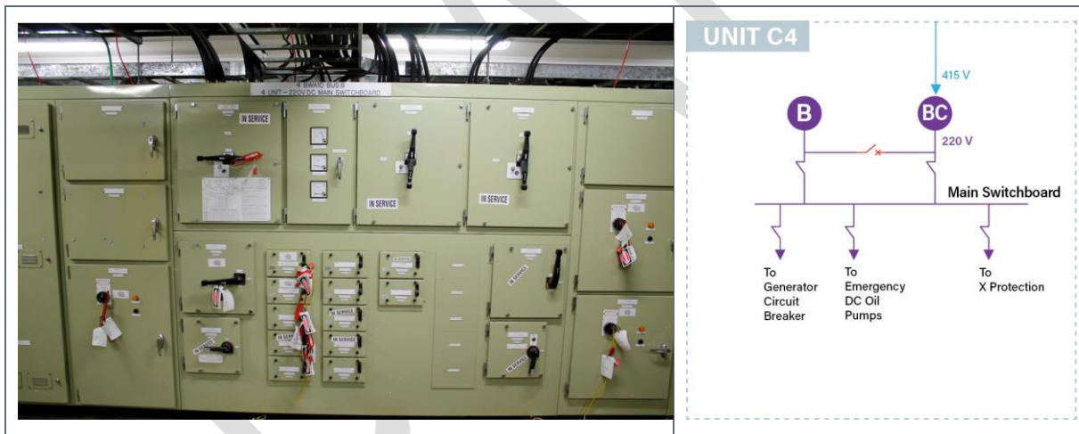
Figure 62 Unit C4 main switchboard
