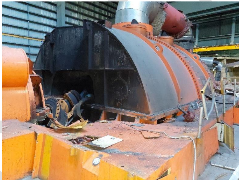
Figure 39 Heat damage to LP turbine casing
