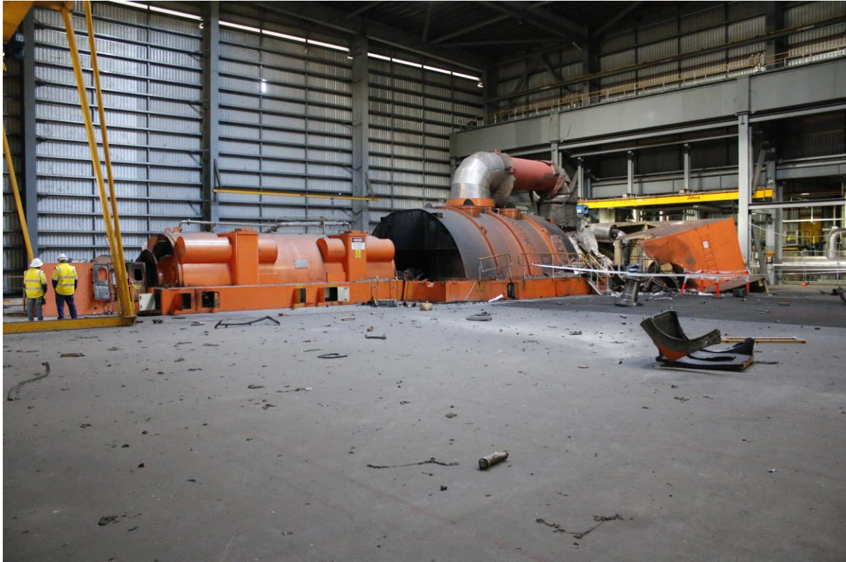
Figure 33 Damage to Unit C4
