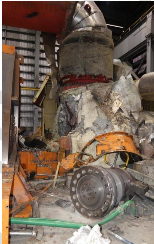
Figure 37 Damage between LP and HIP turbines
