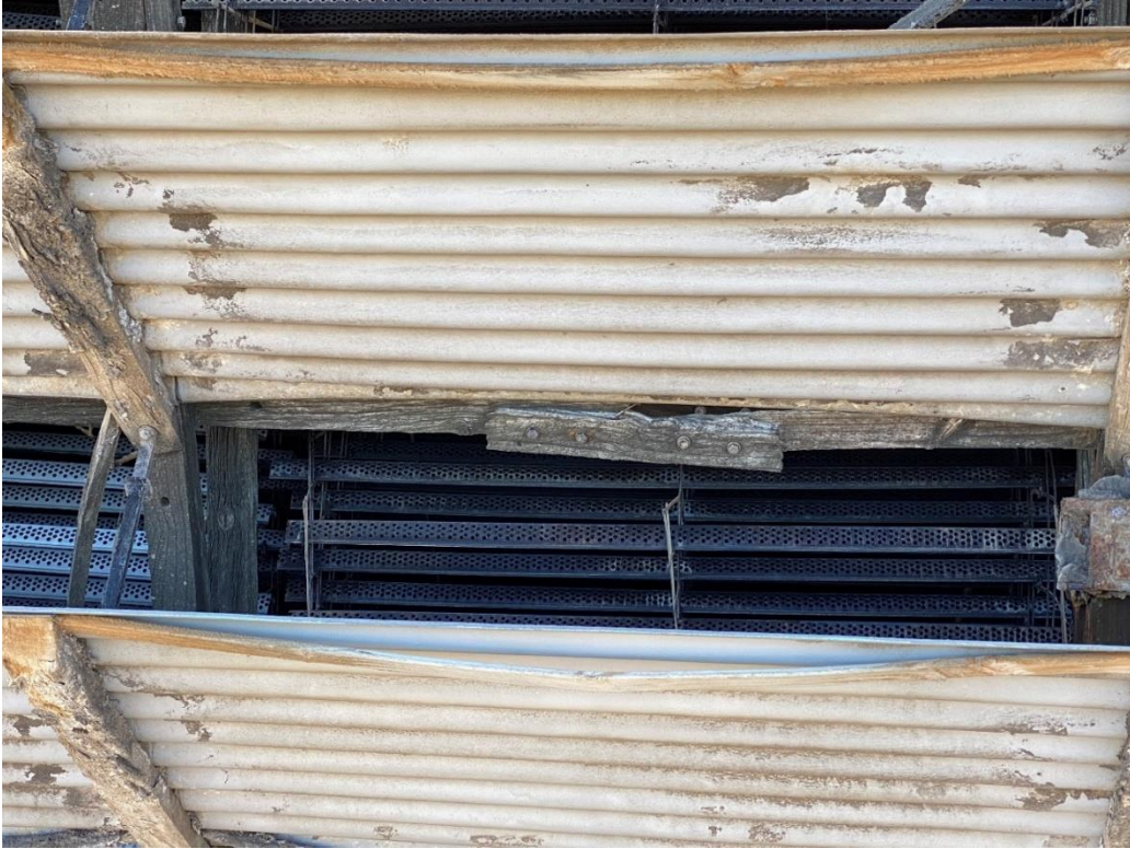
Figure 5.20 Louvre sheet D-mould timber eroded and absent in many locations. Also eroded longitudinal girt and splice
