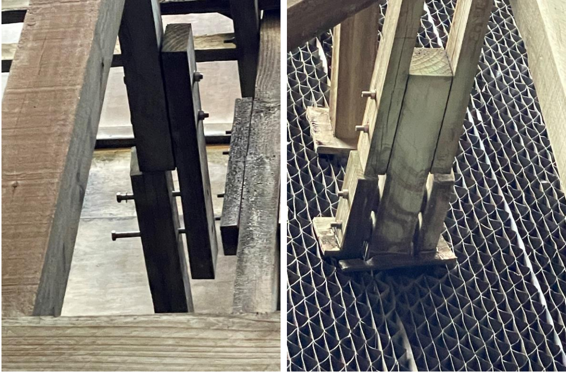
Figure 5.1 Left – Nuts missing, danger of bolts falling out. Right – Loose connection with shear plates disengaged, alternatively these are spacer blocks
