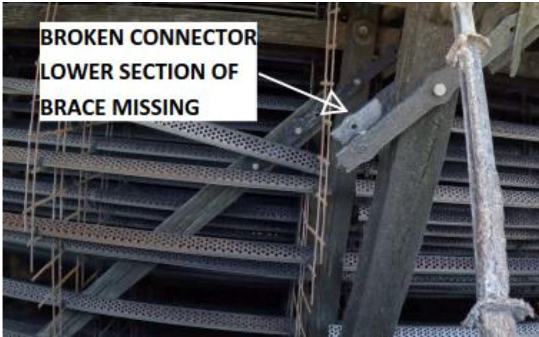
Figure 7.21 Broken Connector and part of brace missing
