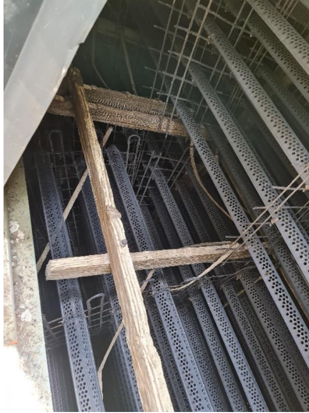
Figure 5.9 Longitudinal girt with chemical erosion
