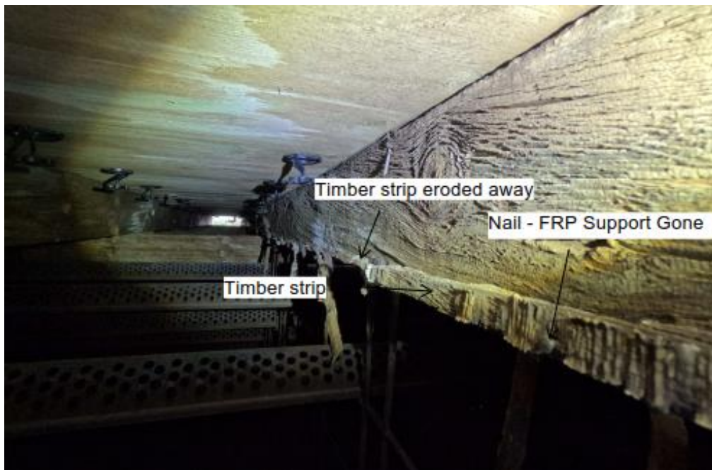
Figure 5.31 Section where the upper fill supports have fallen
