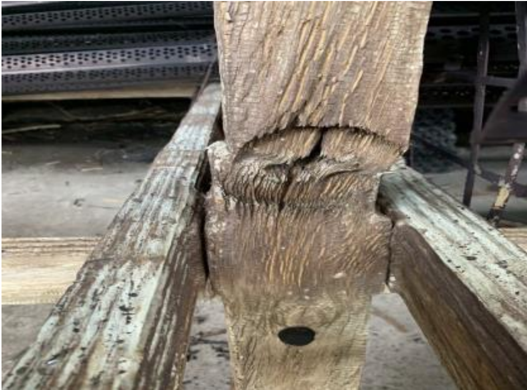
Figure 7.13 Column distortion CT3 location unknown - Marley 2022
