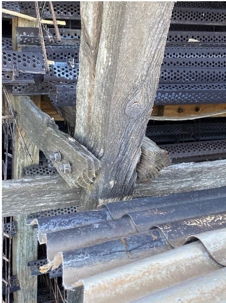
Figure 5.23 Erosion of transverse girts and column. Cut louvre sheet in the foreground
