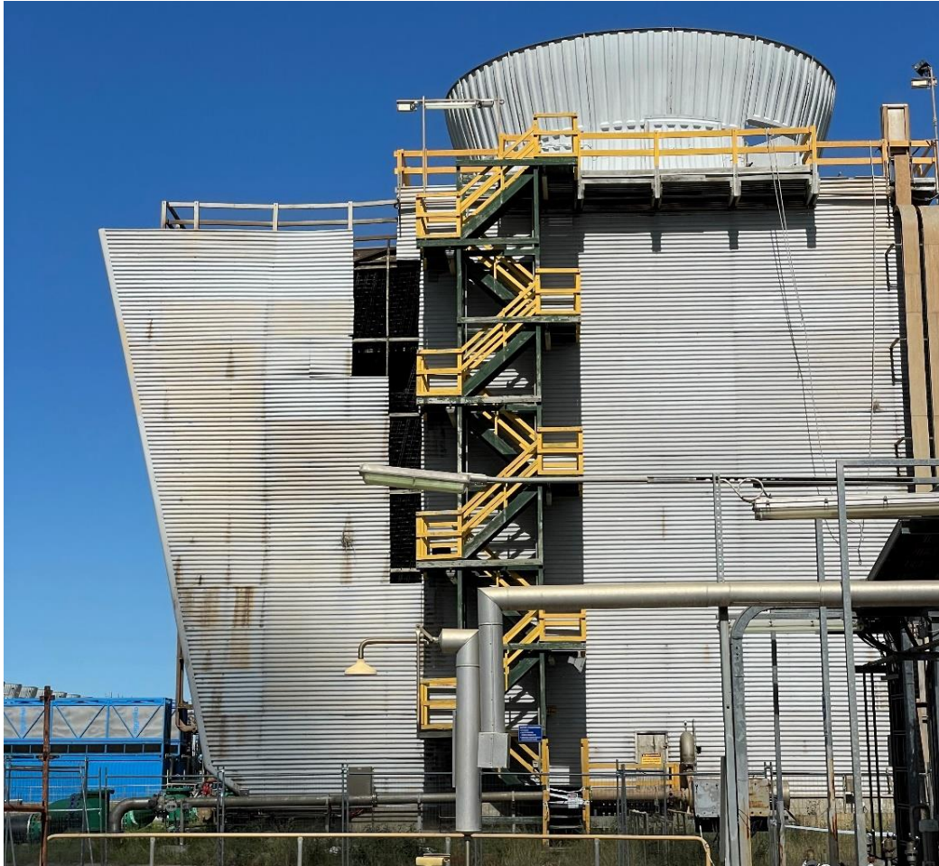
Figure 1.4 Cooling tower CT3 - Cell 1 internal collapse (2022 Photo)
