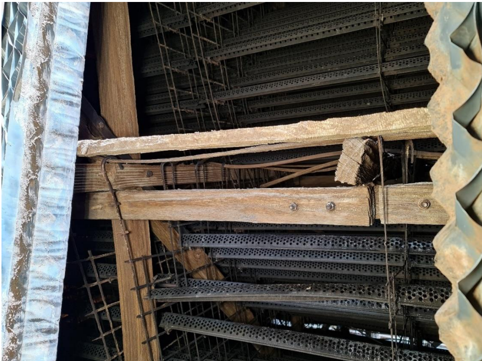
Figure 5.8 Longitudinal girt with chemical erosion. Twisted end of intermediate girt due to bottom fixing only
