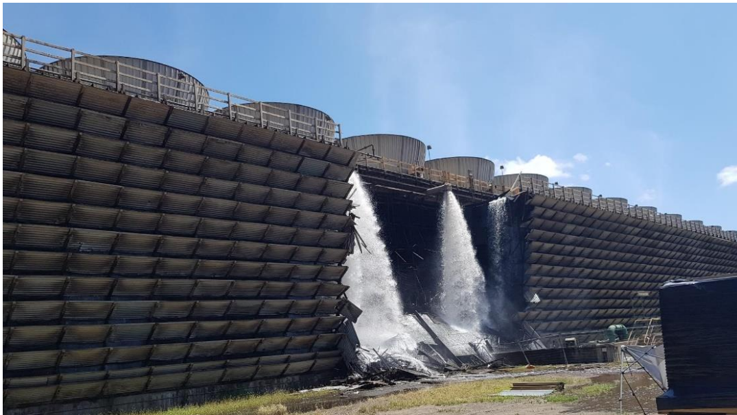
Figure 1.6 Cooling tower CT3 - Collapsed cells 8 and 9 north (2022 Photo)
