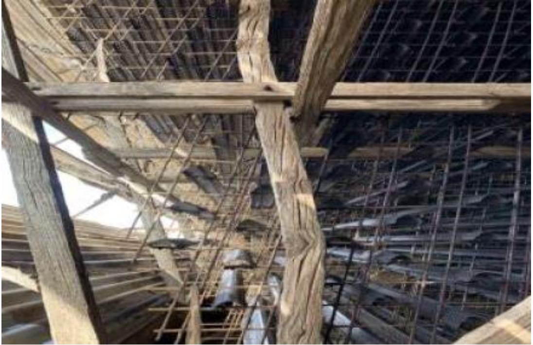
Figure 7.9 Example of column distortion reported throughout wet areas. Note first vertical column adjacent louvre columns - Marley April 2022
