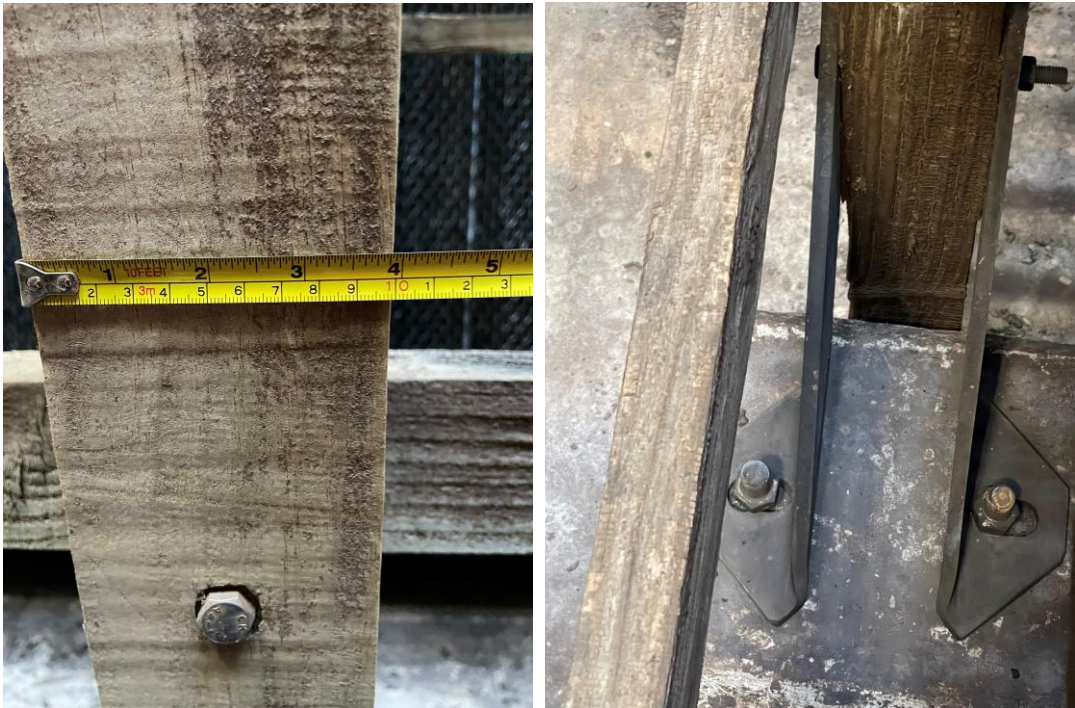
Figure 5.4 Left - No washer or undersized washer penetration. Right Anchor plate with no washers
