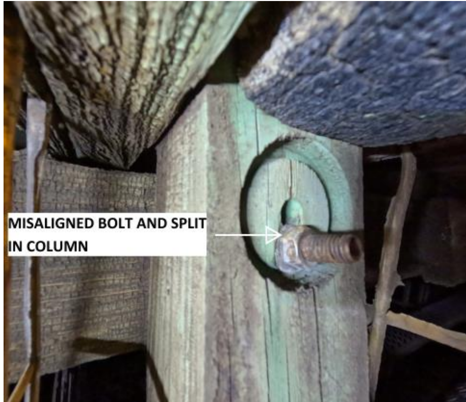
Figure 7.18 Column/Girt bolt misalignment - unknown location
