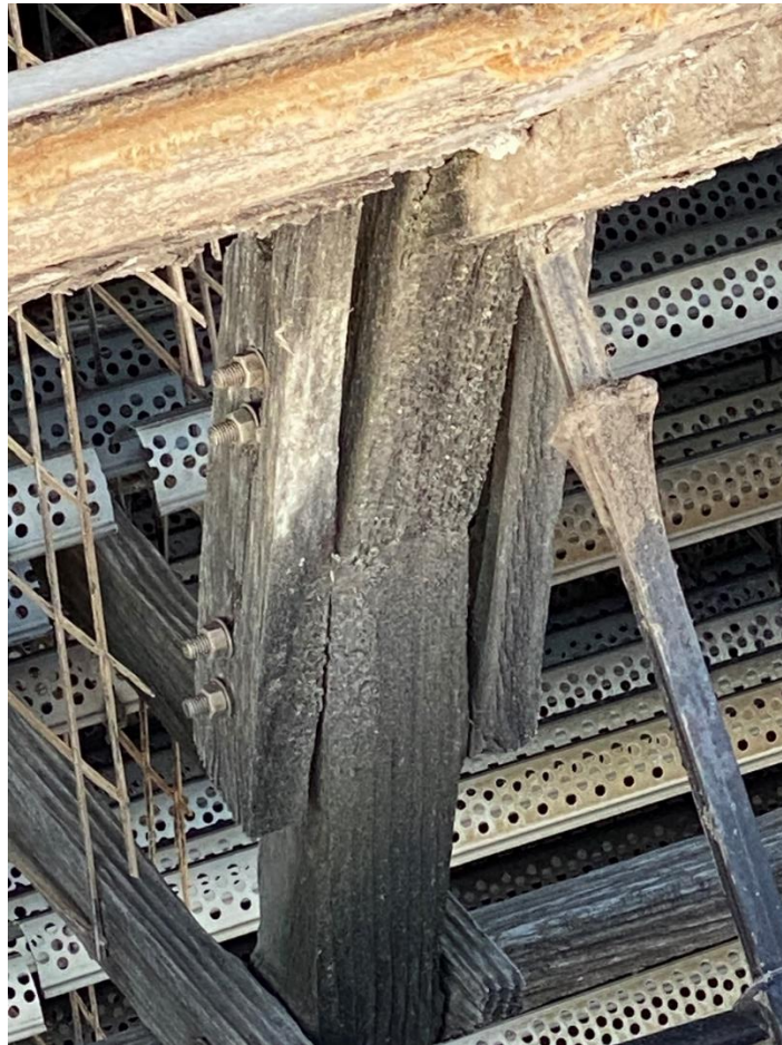
Figure 5.21 Column bent at splice
