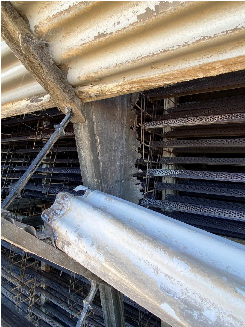
Figure 5.19 Remnant of the cell divide plywood potentially. Loose louvre sheet in the foreground
