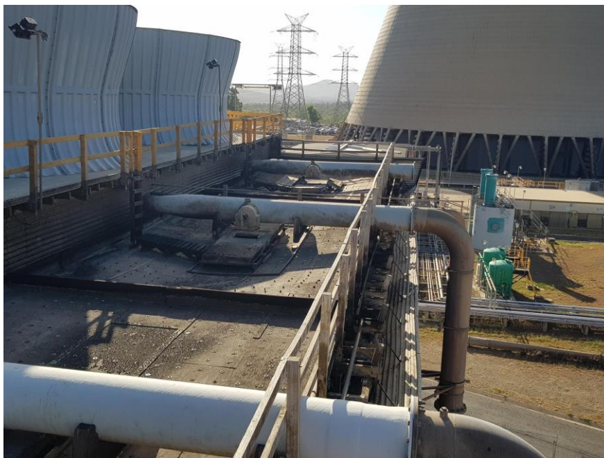
Figure 7.8 Subsidence in hot water basin CT 3 cells 1 and 2 - CS Energy
