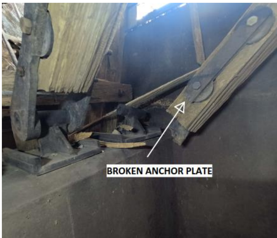
Figure 7.20 Broken anchor plate on a longitudinal louvre brace
