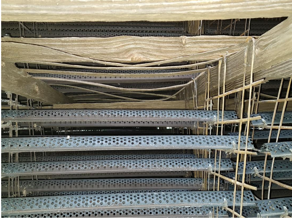
Figure 5.29 Remnants of the D-mould support strips and the staples supporting the FRP grids
