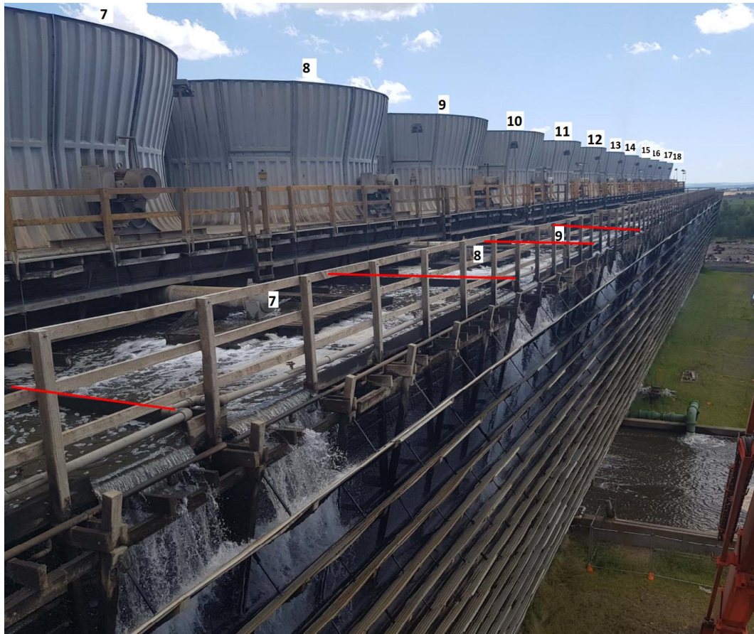
Figure 7.6 Overflow through cut outs in hot water basin
