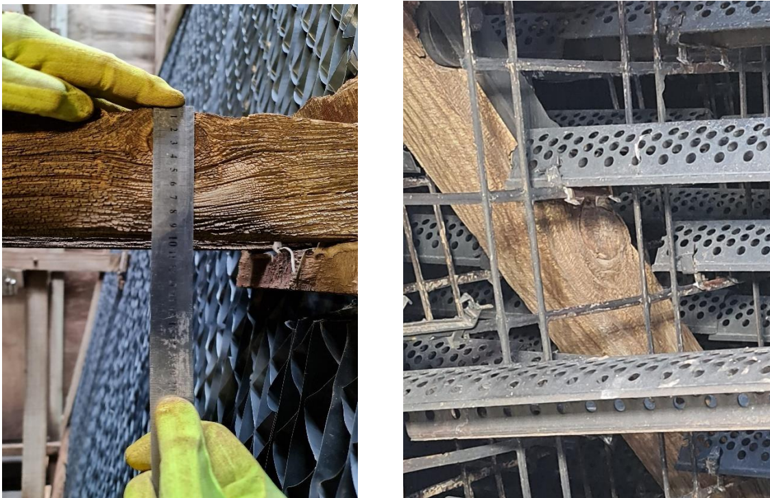
Figure 5.6 Left - Knot in horizontal girt with chemical erosion. Right - Knot in diagonal brace, chemical erosion
