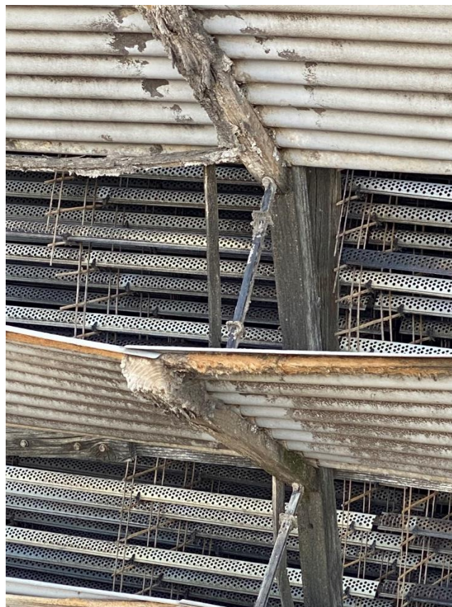
Figure 5.16 Louvre support timber sagging where the FRP plastic tie has come undone
