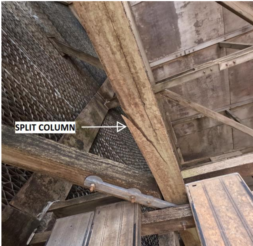
Figure 7.19 Column split in plenum area
