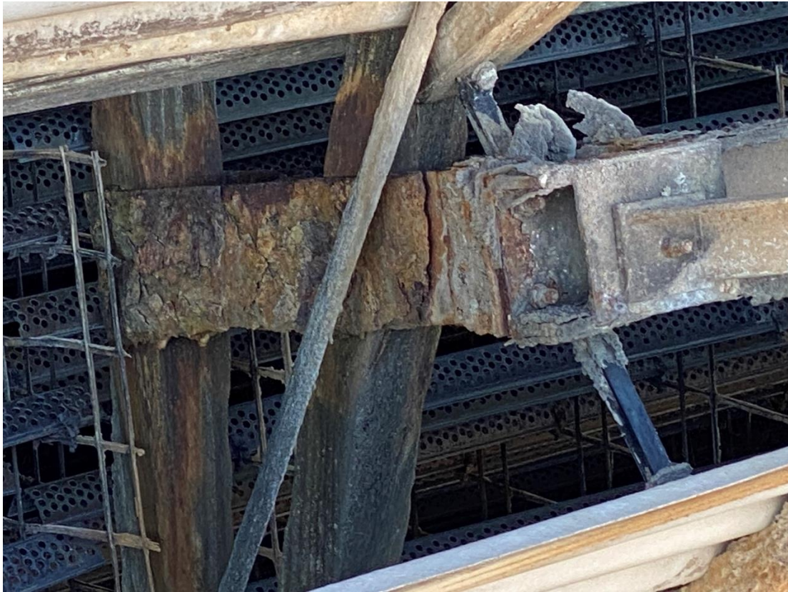
Figure 5.15 corrosion in the riser pipe braces
