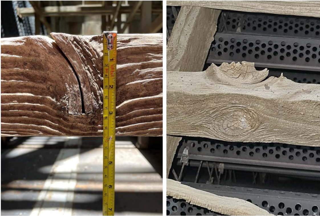
Figure 5.5 Left and Right - Knots in horizontal girts - chemical erosion
