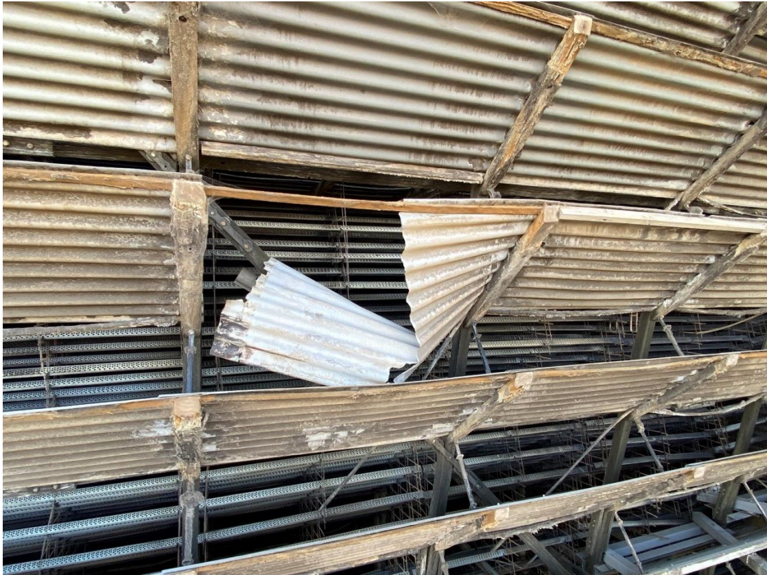
Figure 5.13 Close up of broken louvre sheet - typically damaged sheets were cut and removed
