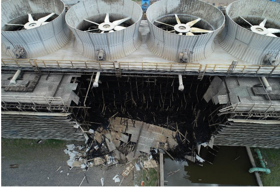
Figure 1.7 Cooling tower CT3 - Aerial view of cells 8 and 9 collapse (2022 photo)
