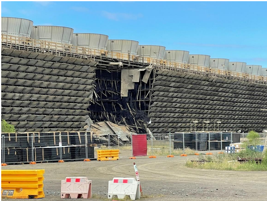
Figure 1.2 Cooling Tower CT3 viewed from the north-east showing collapsed cells 8 and 9
