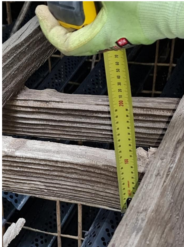
Figure 5.10 Transverse girts chemical erosion, original depth 100mm and 80mm remaining
