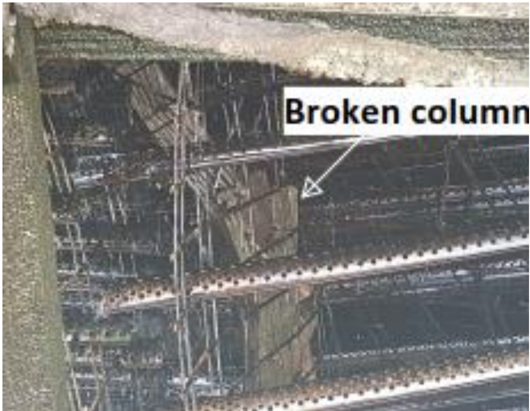
Figure 7.12 Broken Column CT3 Cell 7 - CS Energy
