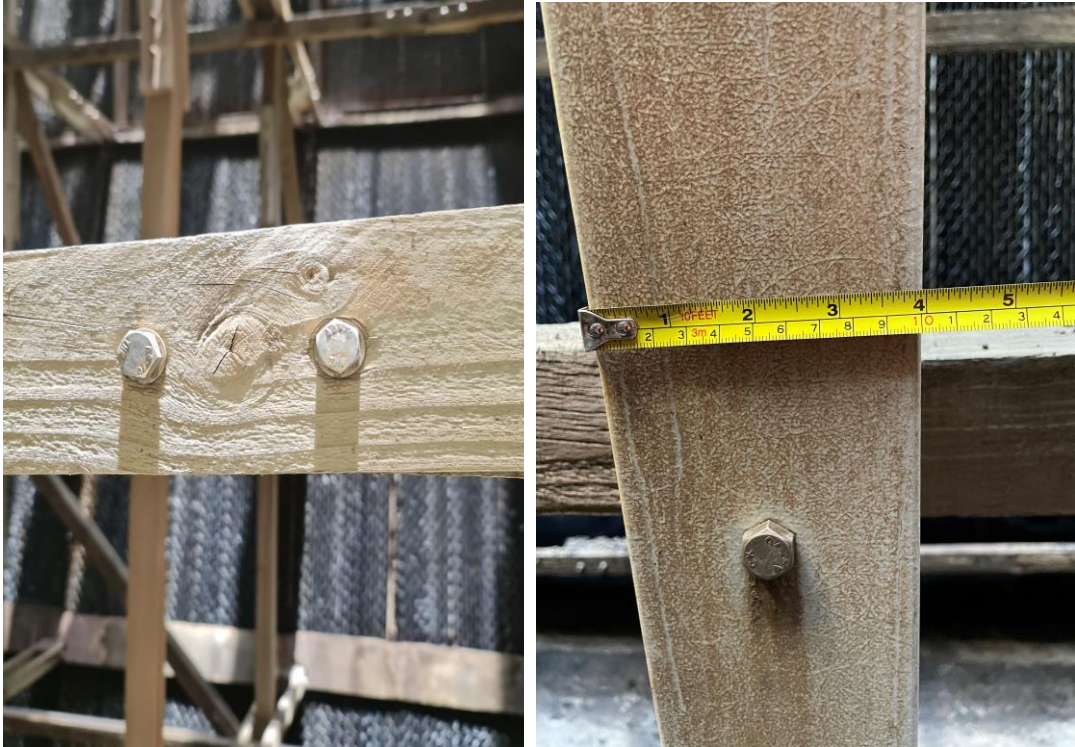
Figure 5.3 Left - Undersized washers. Right: No washer in FRP column
