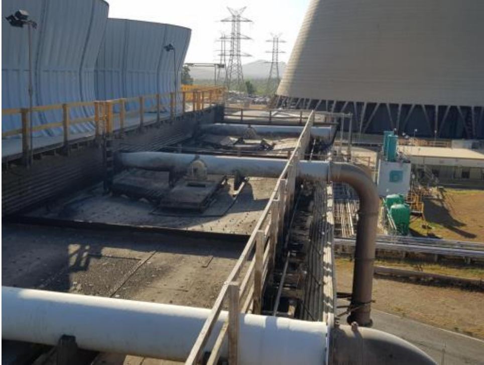
Figure 1.5 Cooling tower CT3 - Cells 1 and 2 hot water basin subsidence (2022 Photo)
