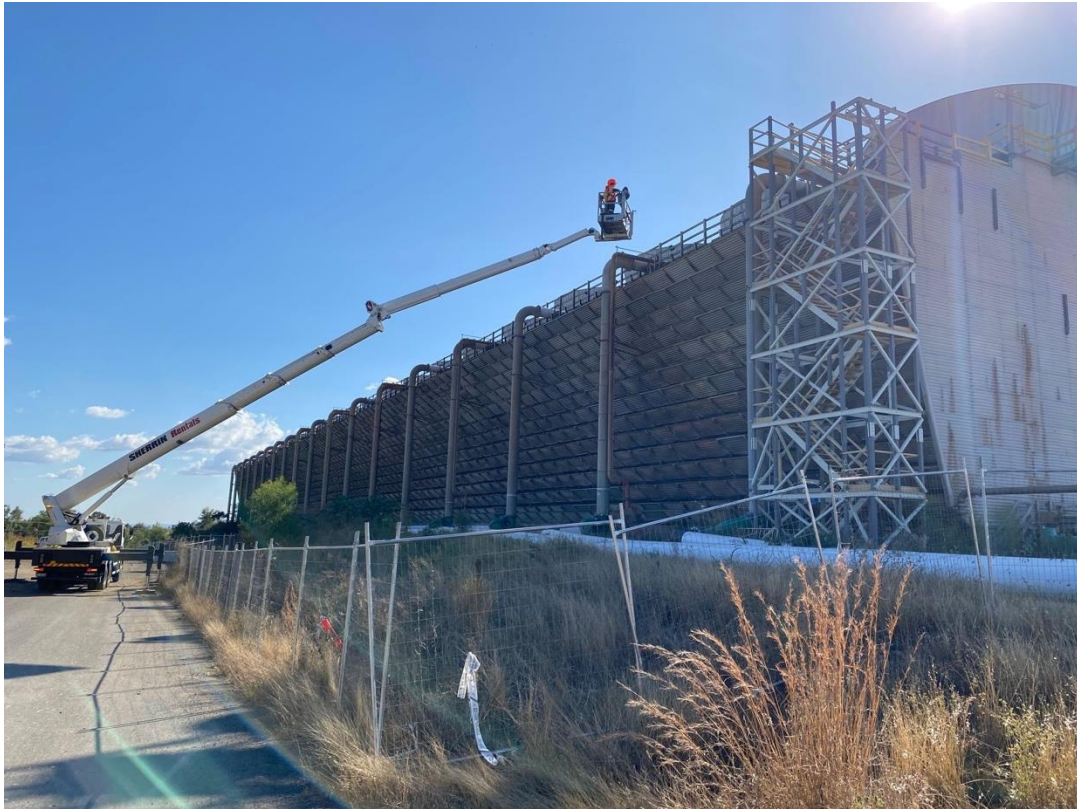
Figure 5.11 The reach of the EWP approaching its limit -South facade of CT4
