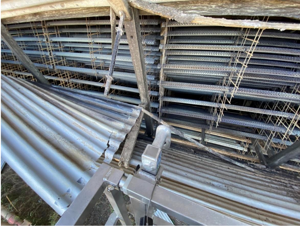
Figure 5.17 Louvre support member that has dropped and FRP tie is hanging free
