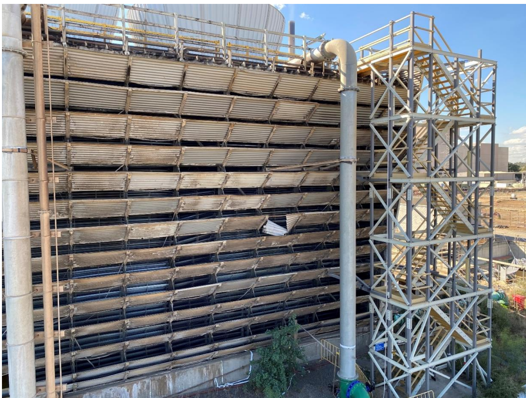
Figure 5.12 Typical damage to louvre sheet
