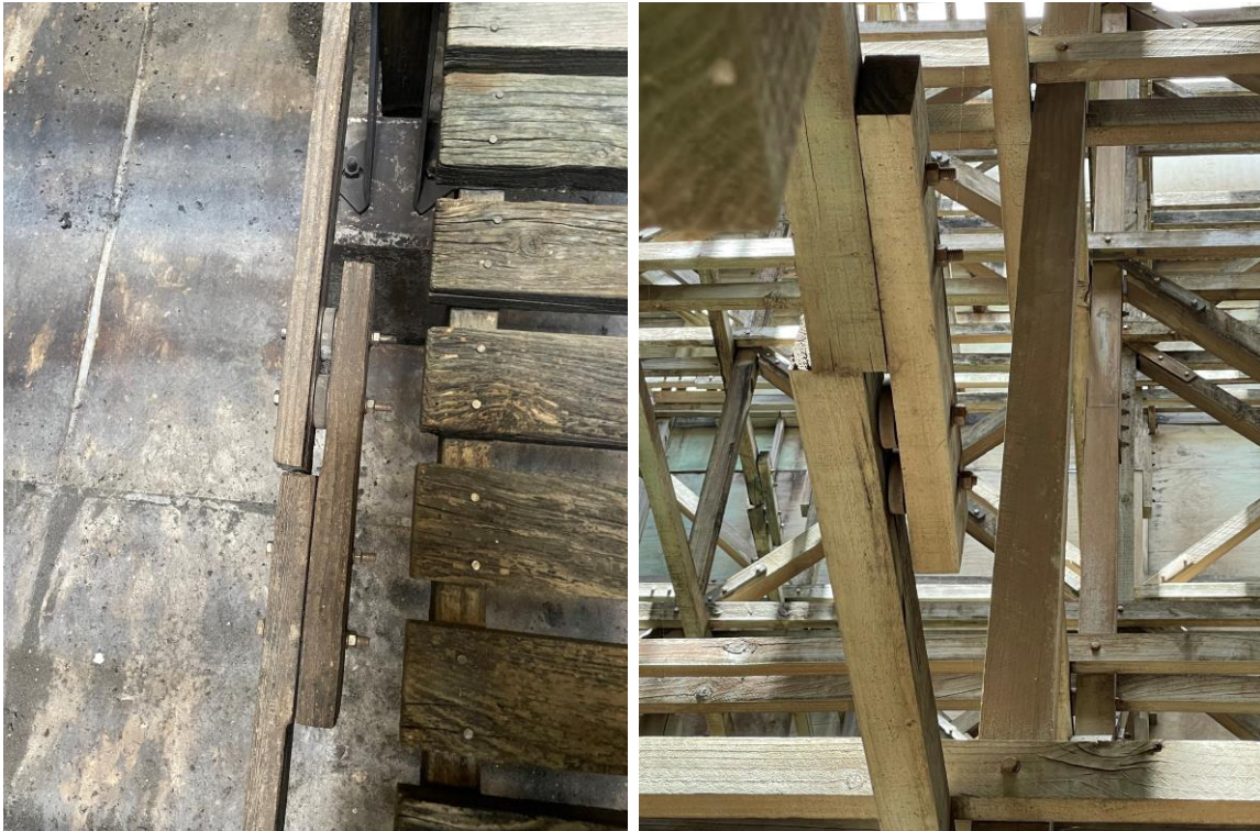
Figure 5.2 Left and Right – Loose connections, misaligned girts with shear plates disengaged, alternatively these are spacer blocks
