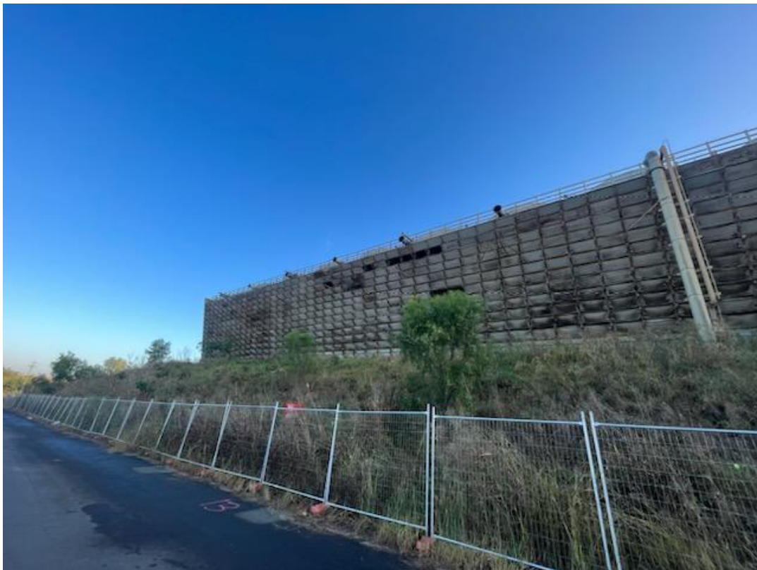
Figure 5.27 Several sections where louvre sheets were removed. Access was granted and riser pipes removed
