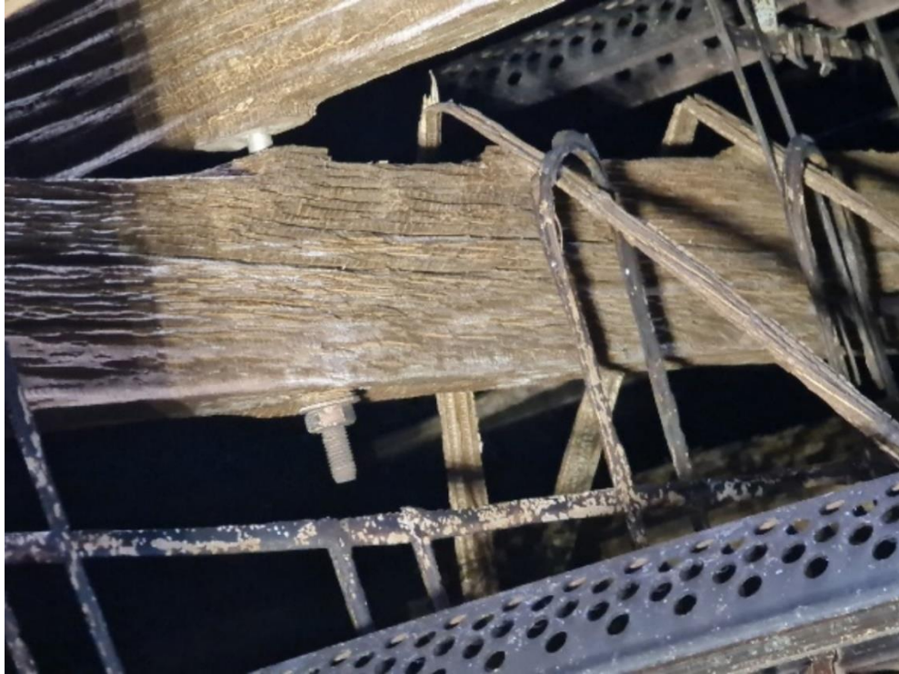
Figure 5.7 Transverse girt with chemical corrosion. Timber D-Moulds completely eroded
